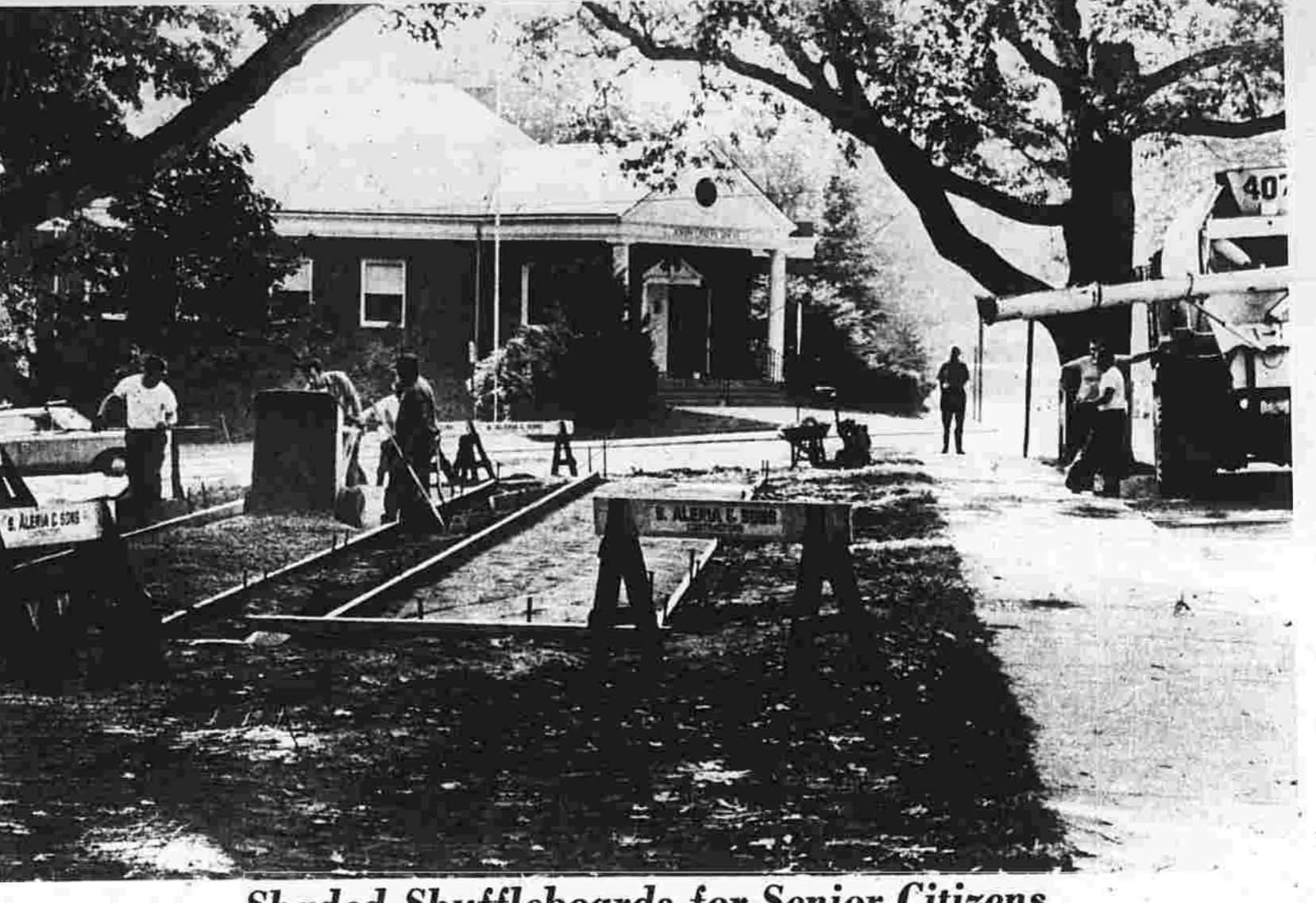
Shaded Shuffleboards for Senior Citizens Shuffleboards are being installed by the Public Works Department across the street from the Senior Citizens Center.
